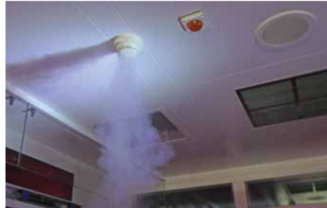
Smoke detector in test ↘
